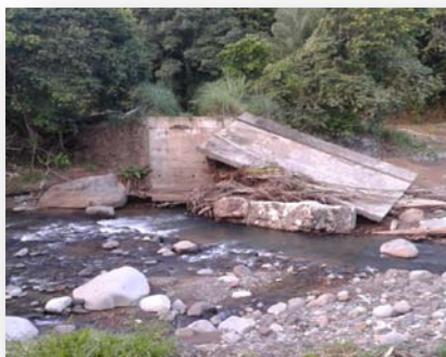
Melville Hall Bridge Failure
