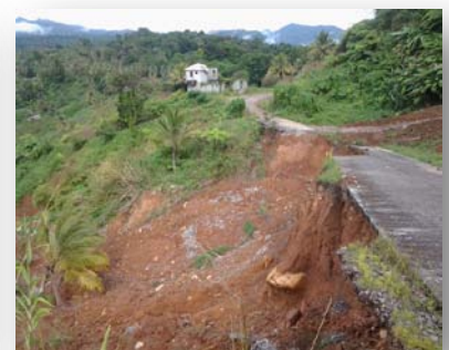
Mero Road collapse
